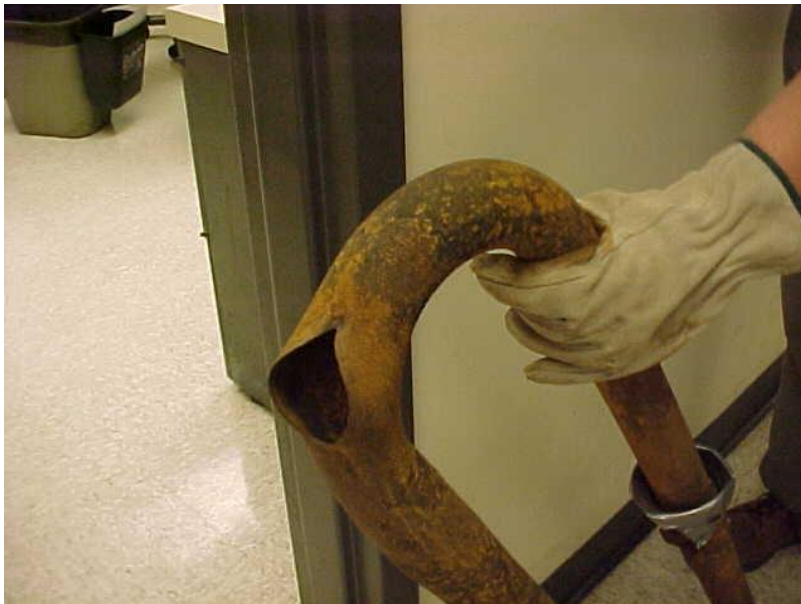
Fig. 3 – Short term overheat failure of Superheater tube
